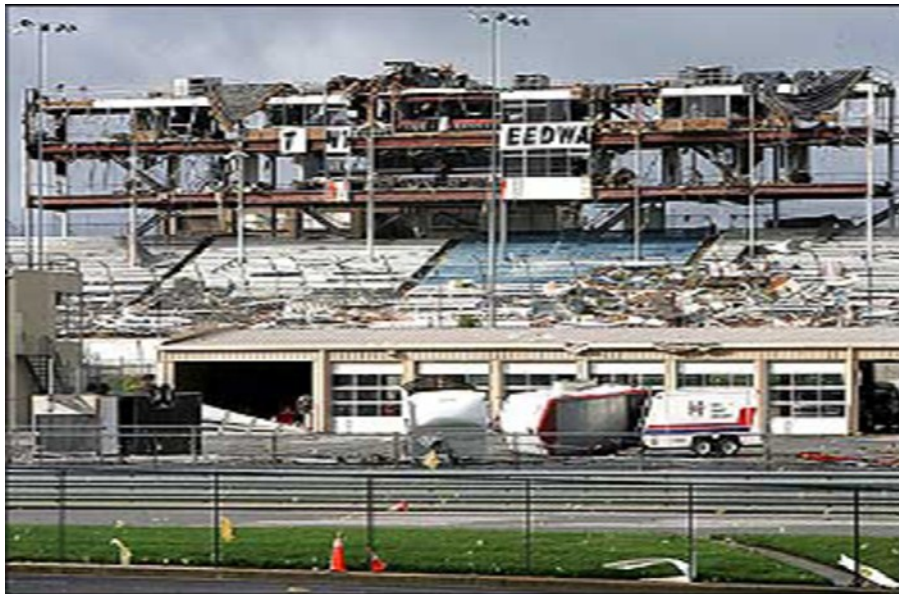
F2 tornado damage to Atlanta Motor Speedway July 6, 2005. Photo by NOAA, NWS Atlanta.
